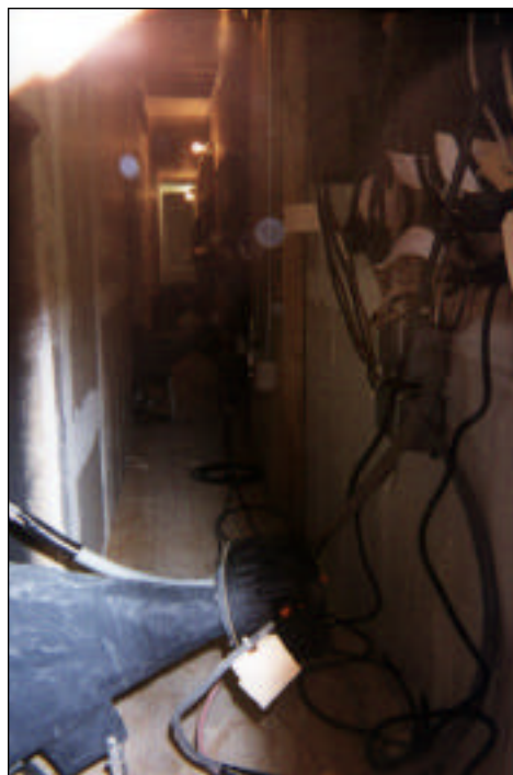
Another view inside of the wall behind the screen at Lucas Film's Stag Theater.
