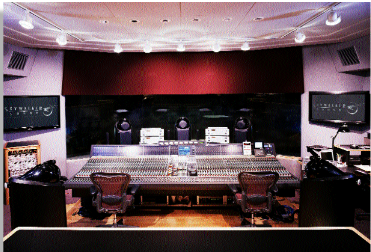
The "B" chain is the Skywalker Scoring Stage Sound Control Room is interfaced using MIT cable technology and Power Conditioning
